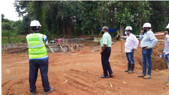
Inspection of hostel construction at the site of upcoming MSME-Technology Centre at Ernakulam on 05.09.2020 by Shri.M.Palanivel, Director I/c, MSME-DI, Thrissur
