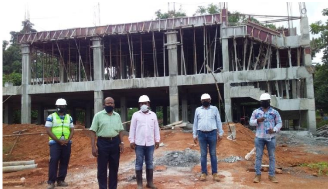
Inspection of canteen construction at the site of upcoming MSME-Technology Centre at Ernakulam on 05.09.2020 by Shri.M.Palanivel, Director I/c, MSME-DI, Thrissur
